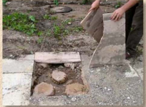
I wonder what caused this breakage??
