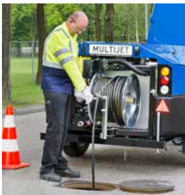
800 litres water on board
