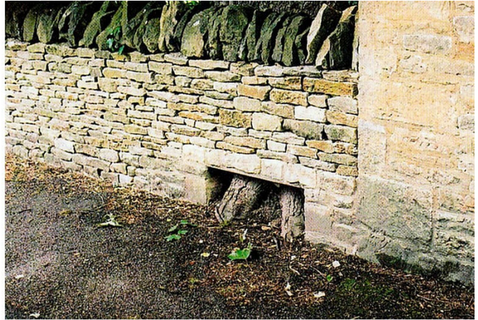
photo - John Roberts [from Tree roots in the Built Environment]
