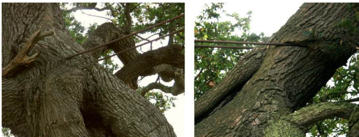
11 Iron bracing rods on the northern stem (left) and on the southern section (right) (Photos Brian Jones 2012)
