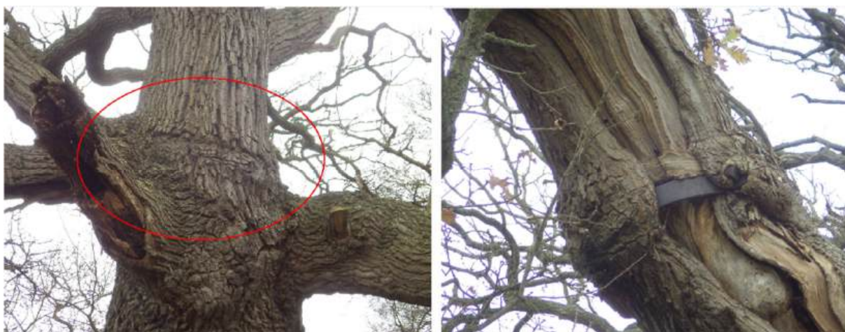
12 Left: Rear of northern stem: the bracket entirely hidden by overgrown wood (ringed) Right: Bracket partly exposed at the rear of the leaning, southerly section. (Photos JPR 2020)
